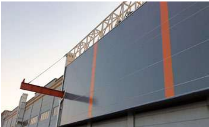
Fold-up door for crane gantry
